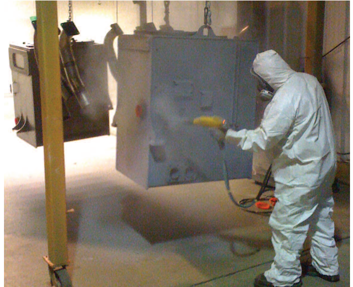
FIGURE 6 – Tank and fill necks manufactured at The IFH Group being powder sprayed.
